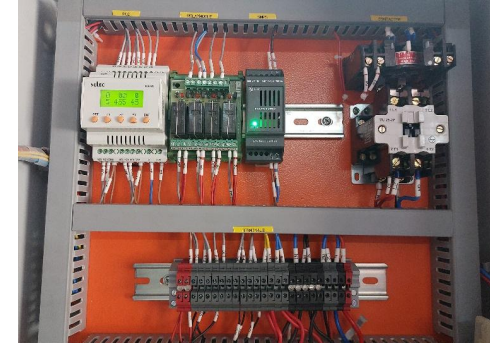
Electric Panel Box
