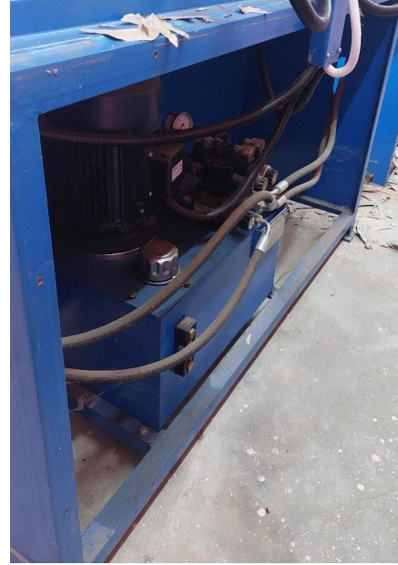
Oil Tank Back Side
